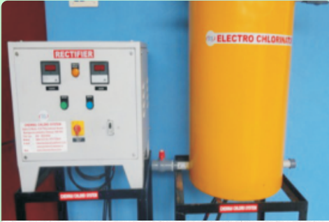
CHLOROGEN - ON SITE CHLORINE GENERATOR
